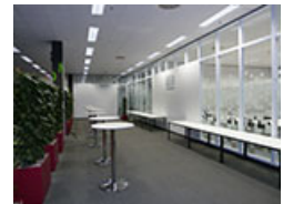
LED office lighting
